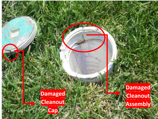
Damaged Cleanout Cap & Assembly
